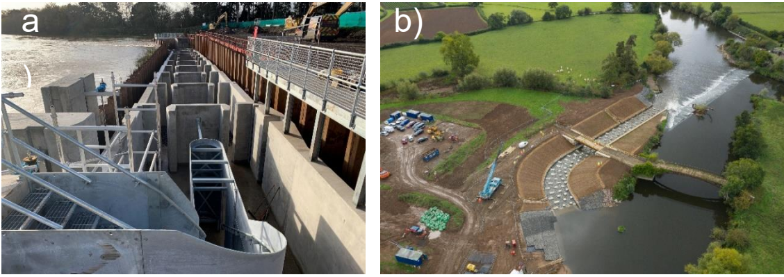
Figure 7.1: Ongoing fish passage remediation efforts in the River Severn catchment. a) Downstream-facing view of ongoing construction of deep vertical slot fish pass at Weir S3 (Diglis, Worcester); b) aerial view of recently-completed bypass channel and rock ramp fish pass at Weir S4 (Bevere, Worcester). Photographs courtesy of a) Charles Crundwell and b) Skynique DGI.
